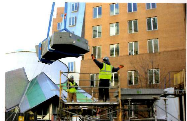
Figure 1.10 The fabrication and installation process required an intense interaction of man and machine as blocks were cut, measured, finished, handled, set, and placed.
